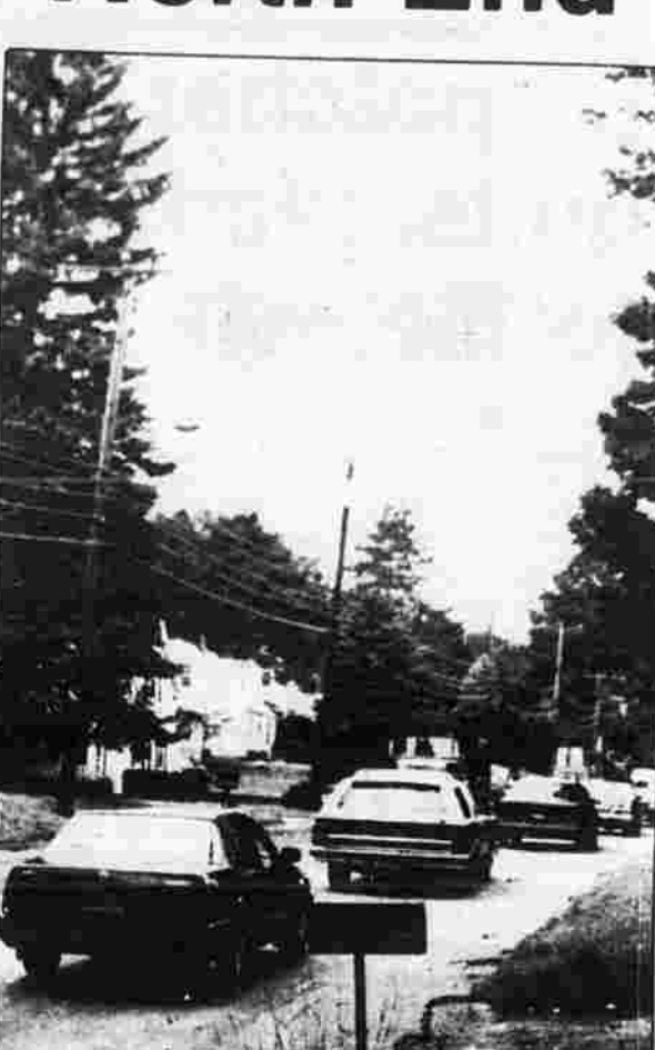
SLOW GOING — These cars were backed up on North Main Street one afternoon this week because of the installation of a sewer. The sewer project is one of several in progress in the North End of town which has slowed traffic there. David Hulme, a Union Street resident, says he is concerned about access for emergency vehicles, but town officials do not share his concern.
